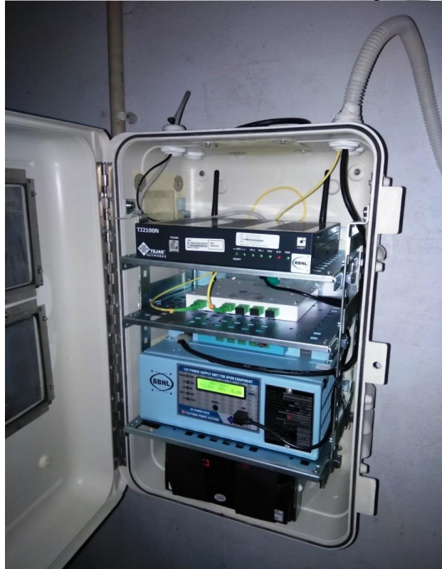
Fig 5.3. Image of ONT, CCU, Battery installed at Gram Panchayat
