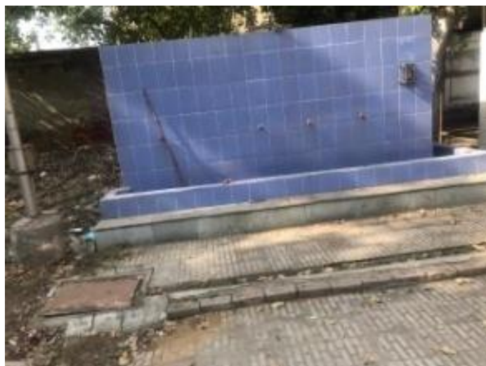
Poor facility of drinking water- Govt school
