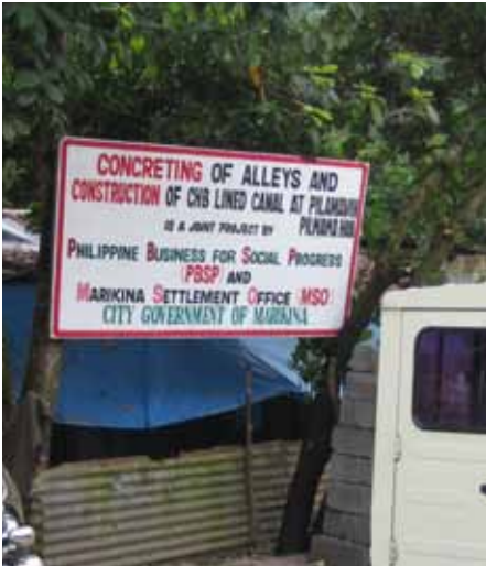
Marikina, Manila: Construction of alleys and footpaths financed under the STEP-UP project Source: F. Steinberg.
