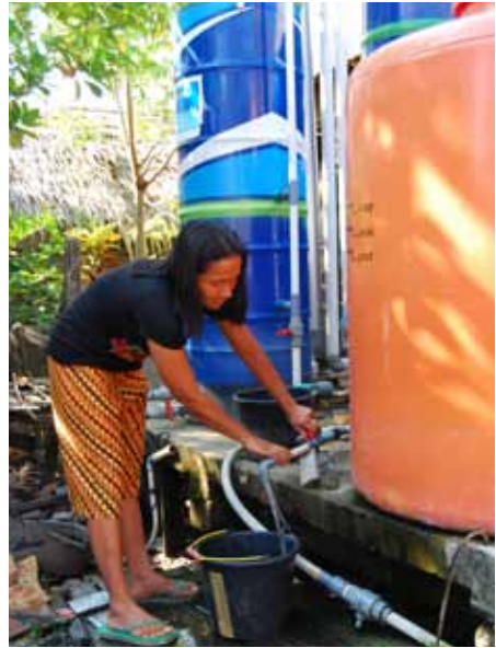
NUSSP community water supply Source: Ministry of Public Works.
