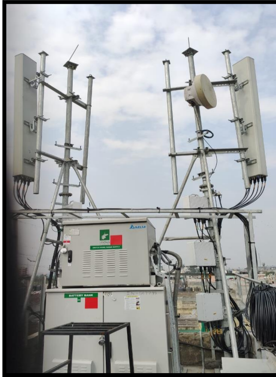
Figure 5.5 : Roof Top Pole (RTP) Site
