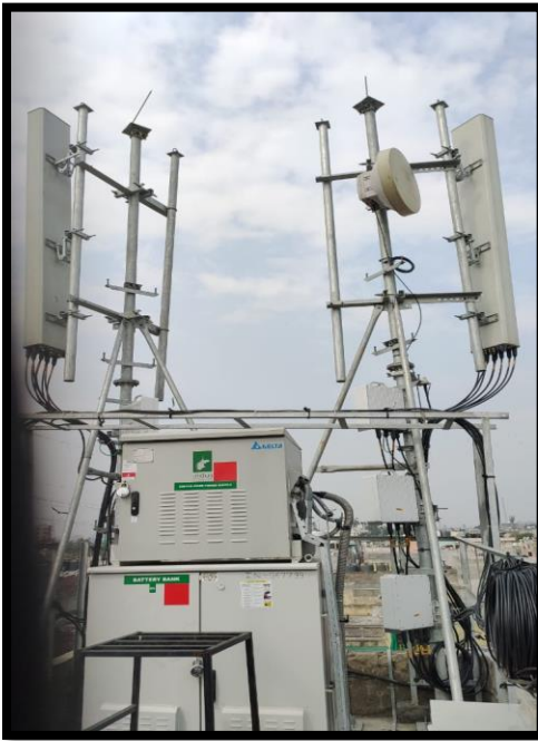
Figure 2.6: An Actual Roof Top Pole Site
