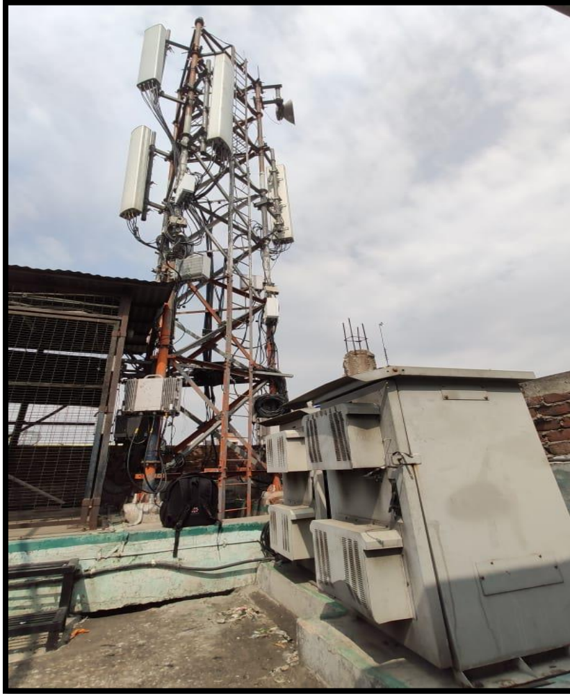
Figure 5.4: Roof Top Tower (RTT) Site
