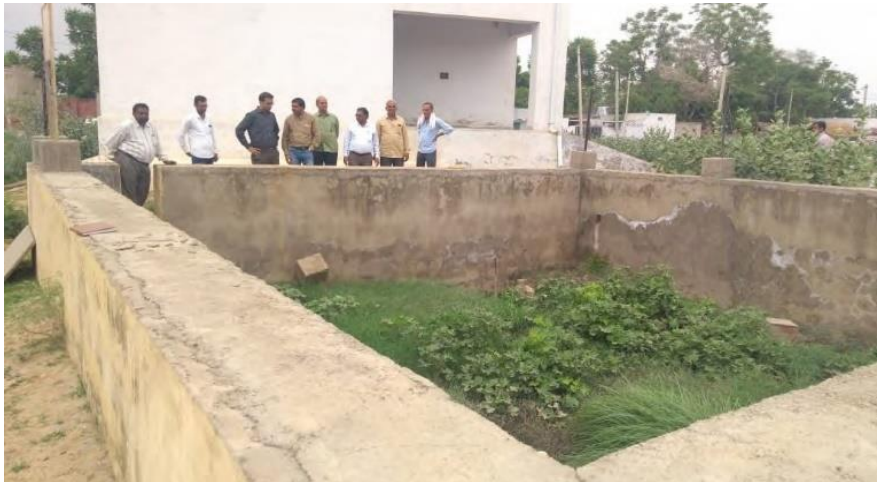
Photo : Dry Well with New Greywater Recharge System
