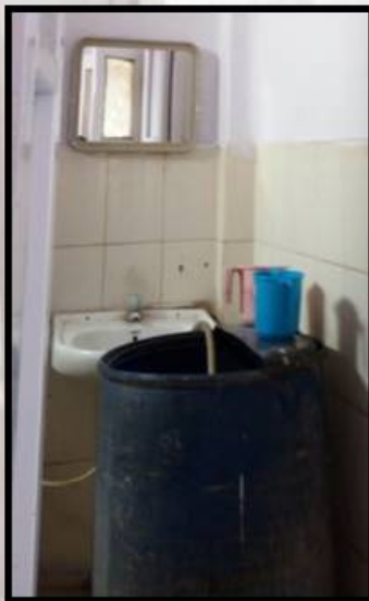
HPO , Mysuru No Proper Water Supply, this tank is used to store water
